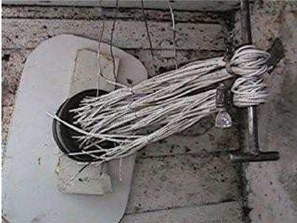
FIGURE 3 - CABLE BUNDLES OVER FUEL CUP LOCATED IN THE EE-BAY
