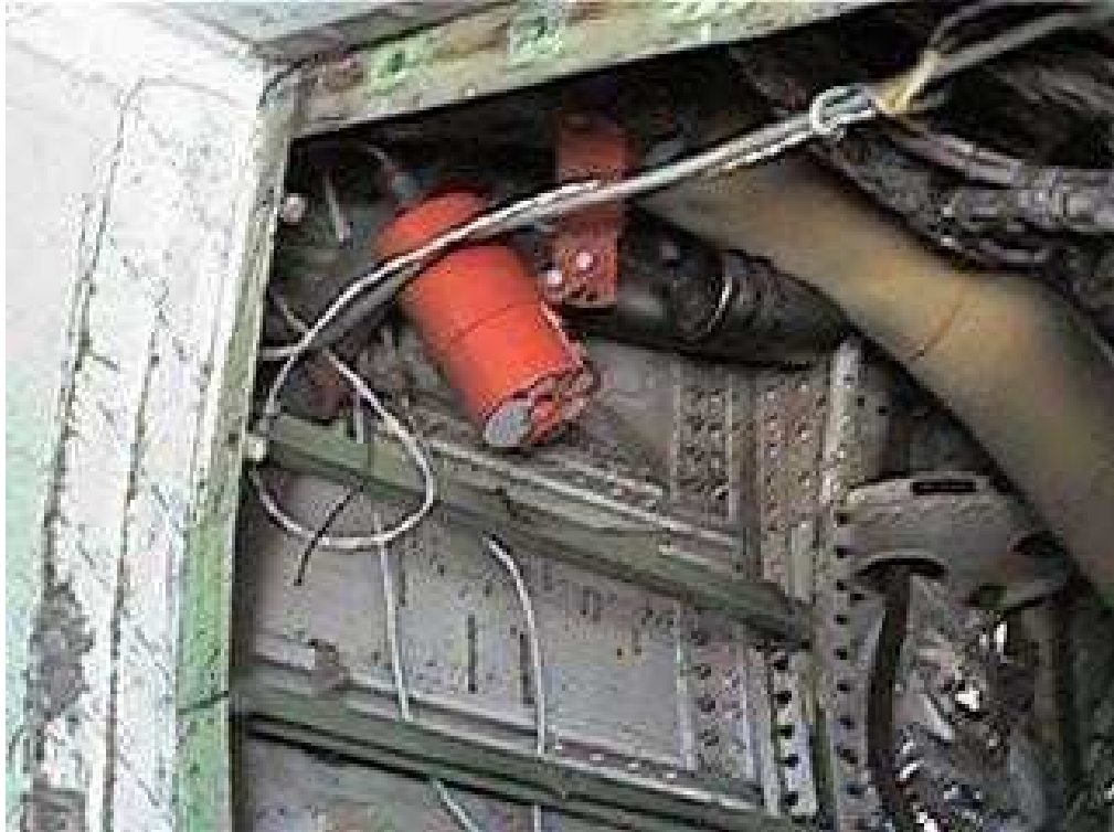
FIGURE 5 - PYROGEN MAG-3 GENERATOR WITH UNINTRUSIVE MOUNTING INSIDE THE EE-BAY
