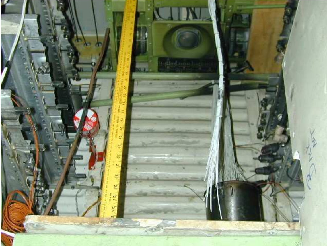
FIGURE 6 - LAYOUT OF THE PYROGEN AEROSOL GENERATORS INSIDE THE EE-BAY AND RADOME AREAS
